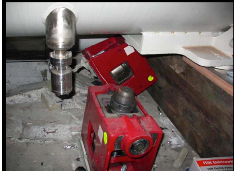
support jacks ripped out of concrete socket
